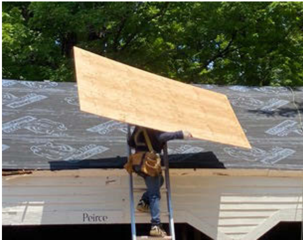
Carrying a 4'x8' plywood sheet up a ladder to cover the first layer: Rhino Roof U20 synthetic underlayment to ward off moisture.
