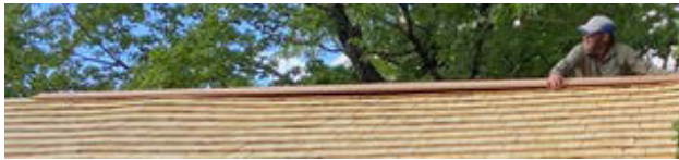
3:12 p.m. With front shingling finished, Harry sets the ridge cap. The flexibility of wood was evident: when the ridge line dipped, the wood was sat upon to make it tight to the shakes. By 4pm the ridge cap is finished and by 4:20 the workers are cleaning up.
