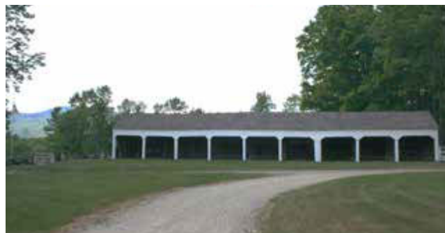
6/21/20 The Horsesheds before new roof.
