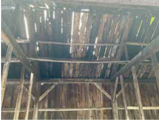
9:45 a.m. Looking up to the sky from inside. Despite gaps, the boards were better than expected, ready for strengthening with 1/2" plywood.
