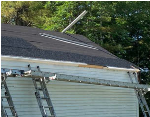
The metal drip edge, a finishing touch, is attached after Cedar Breather and new wooden fascia molding.
