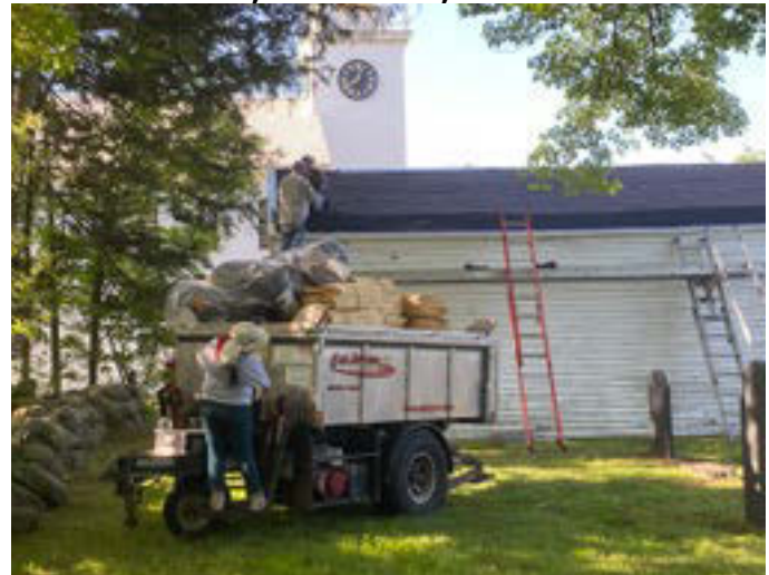
8:02 a.m. Loaded up with cedar breather and shakes to install above the black felt.
