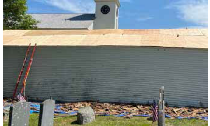
2:00 p.m. Full plywood on both sides, ready for 3 rd layer, black 30-lb. roofing felt, completed by end of day.
