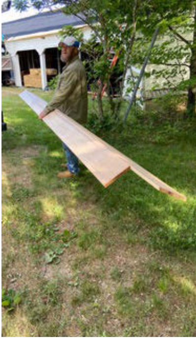
8:00 am Harry carries red cedar ridge cap – two glued parallel boards, each extending an end to avoid having a cross seam that could leak.
