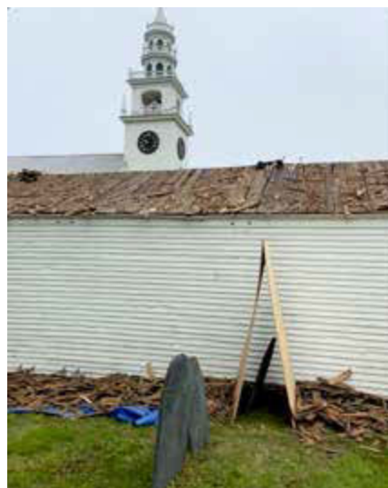
9:40 a.m. 2200 sq. ft. of shingles stripped in 100 minutes; plywood protects 2 nearby gravestones.
