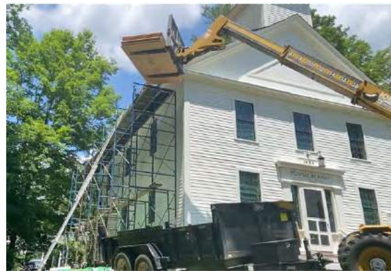
Half inch plywood is taken to the roof by the lift at 1:20 PM on June 29. The west side of Melville's roof was finished July 1 before torrential rains arrived the next day.
