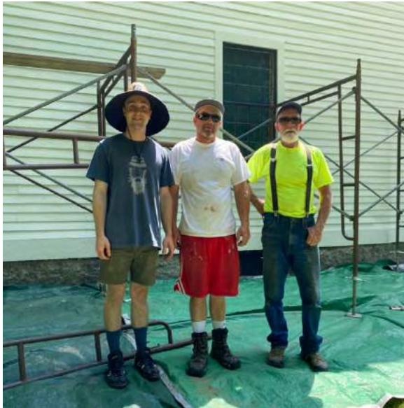
Greg stands between his brother Sam to the left and Jim, his father, to the right, as they begin to put scaffolding up on the west side of the building.
